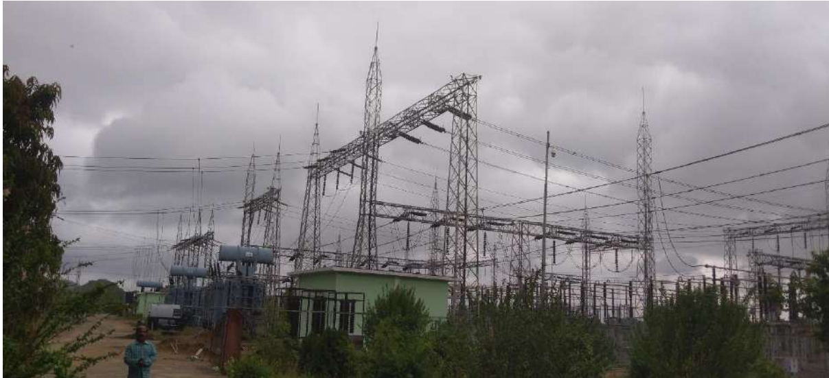
220/132/33 KV Grid Substation, Katapali
