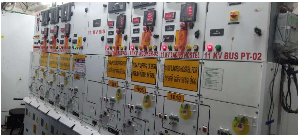
11 kV feeder panels
