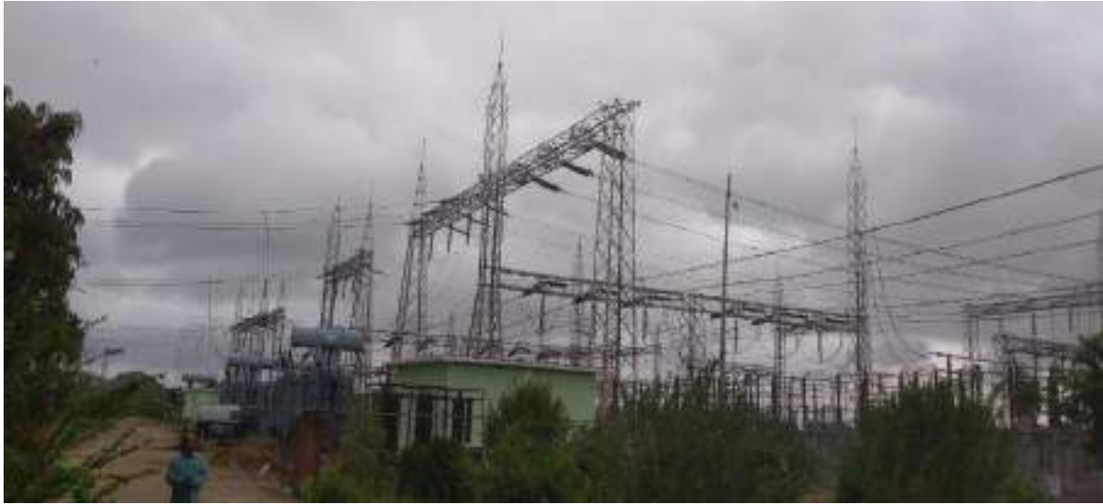
220/132/33 KV Grid Substation, Katapali
