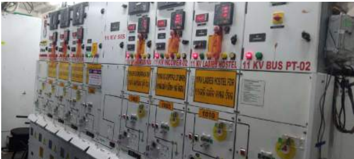
11 kV feeder panels
